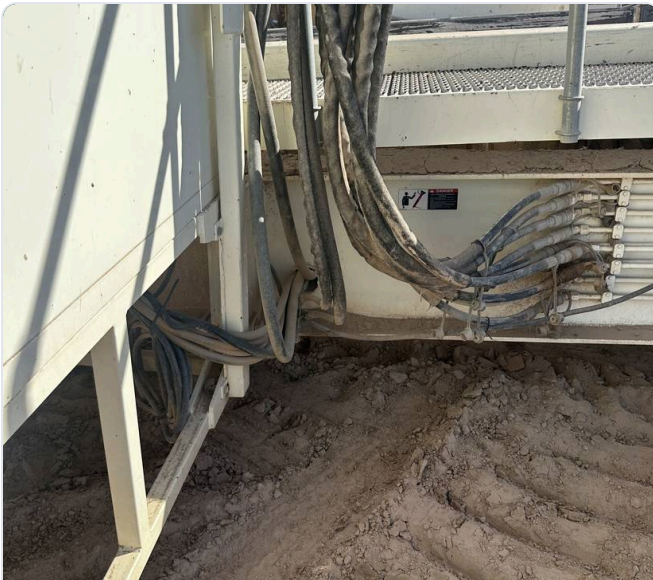
The trench by the power unit. The genset light wiring follows this path.
