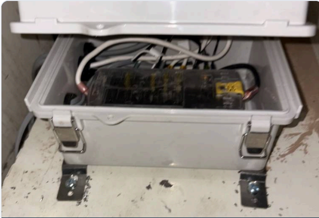
Fuse panel bolted down. The on/off switch is on top.
