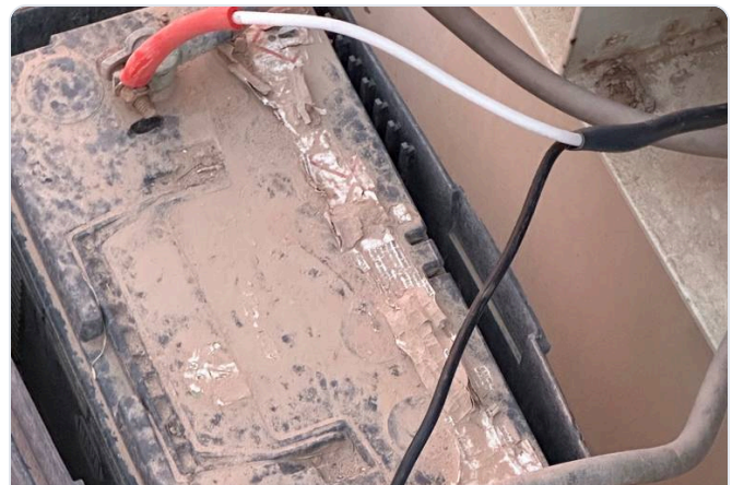
Box leads on the battery. Red to positive, black to negative.
