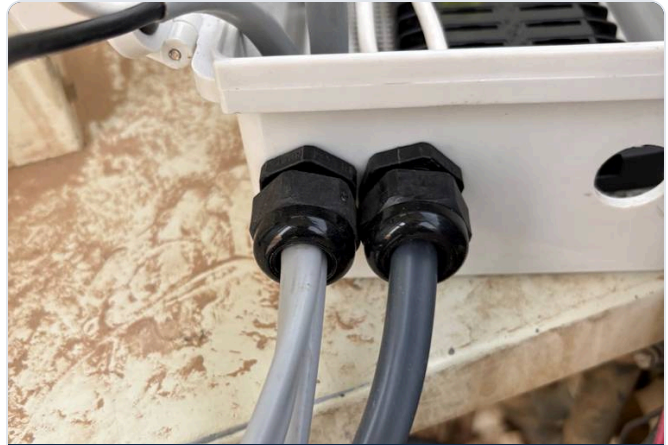
Wires leave the panel through the sealed fittings on the bottom.
