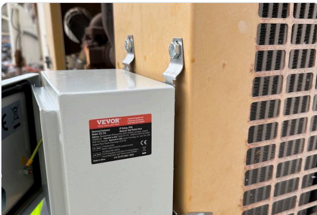
Metal box bolted to the genset, close to the battery.
